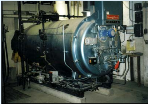
Fire Tube Boiler
